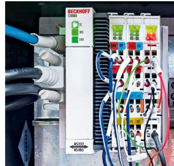
A platform consisting of an Embedded PC (shown here: CX8080), TwinCAT automation software and EtherCAT Terminals controls the semiconductor production for photovoltaics.
