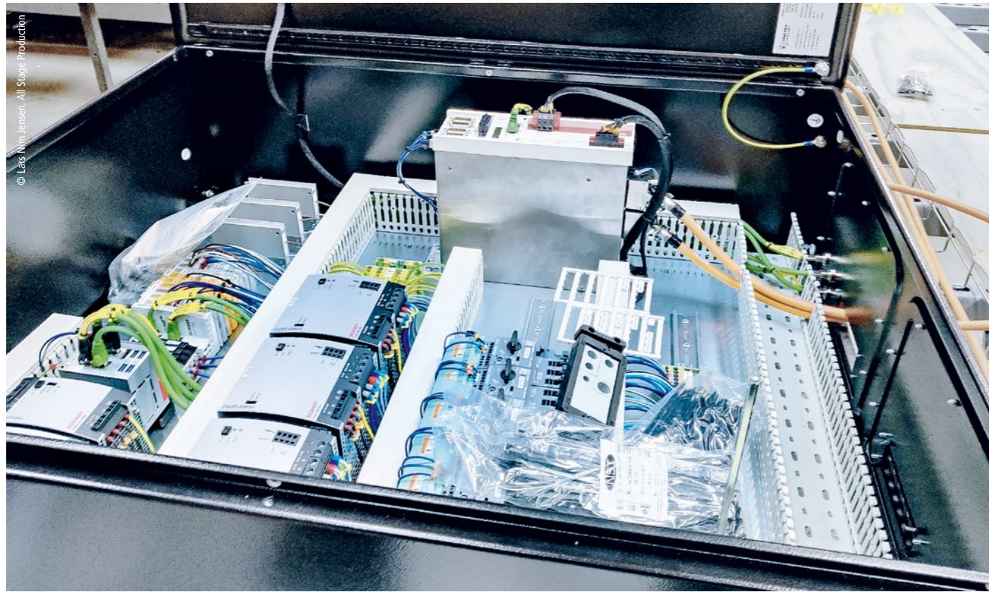
Control cabinet during assembly with a two-channel AX52xx servo drive, a C6017 ultra-compact Industrial PC, and several PS3000 power supply units for the AMI8100 distributed servo drives
